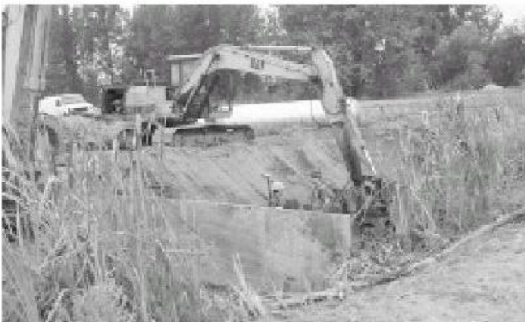
The building of the meandering swale and the earthen dikes where performed using heavy equipment (Port of Portland website).
